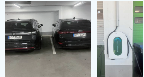
Company Electric Vehicles and Charging Piles
