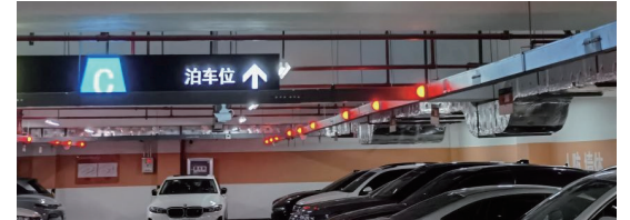
Smart Parking Lighting Fixtures
